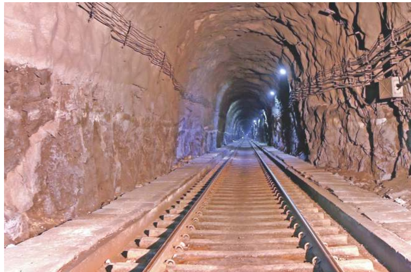
Ballast-less track in Karbude tunnel
