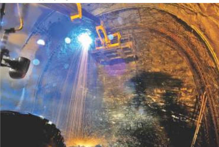
Support fixing in Tunnel T49
