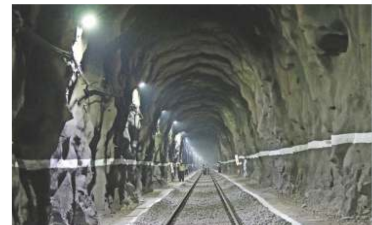
LED tunnel lighting
