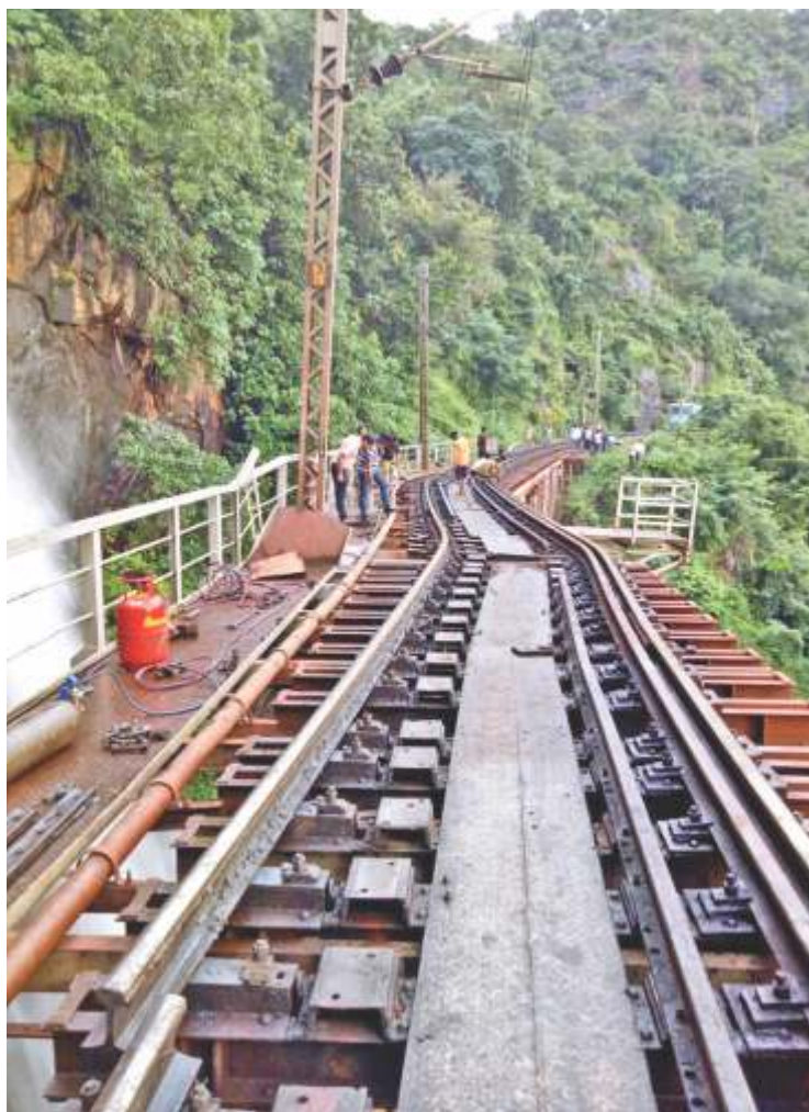
The dislodged rail lines
