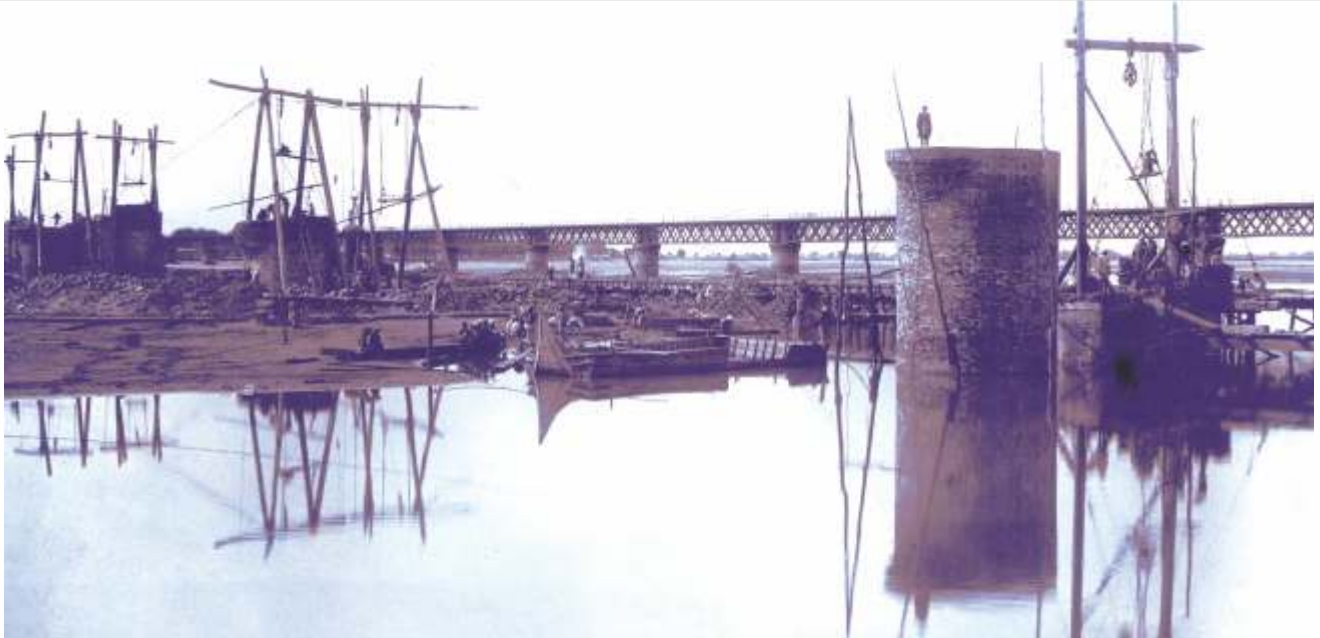
A new bridge was constructed on the Sutlej at Phillaur to facilitate double line working. The work of constructing the piers can be seen in the photograph, taken in 1909. Note the rudimentary means used for construction. The old bridge is in the background
