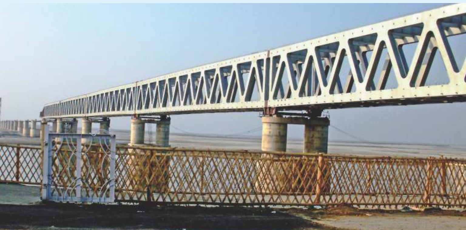
▼ The Bhogibeel bridge pictured in February 2015, when girdering was in progress. The bridge is likely to be opened in 2018
