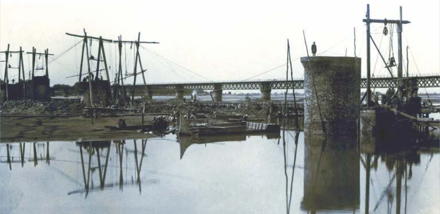
▲ Work of constructing the piers of the new double line bridge. The old bridge can be seen in the background
