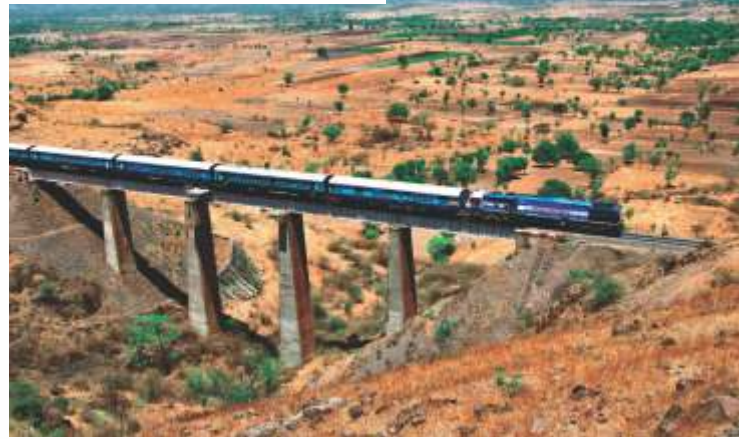
At the end of the cuttings is the second longest viaduct, No. 8, of the section
