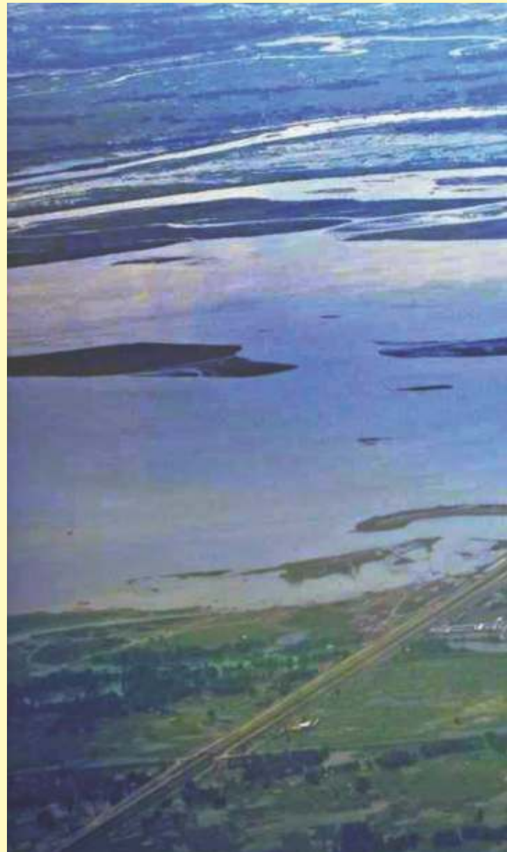
▼ An aerial view of the Bhogibheel bridge at the stage when piers were under construction
