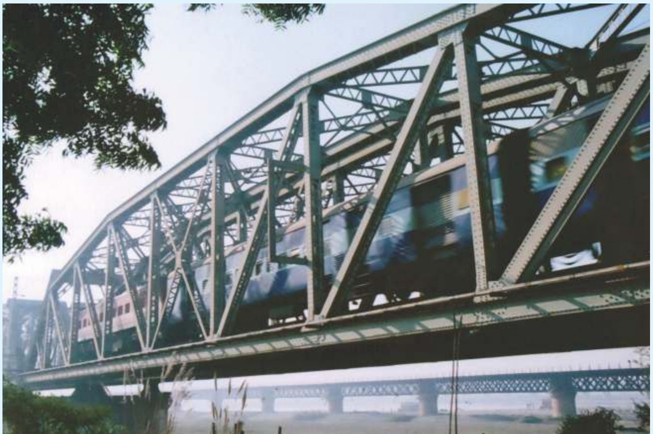
▲ A recent view showing an electric hauled express train passing over the bridge
