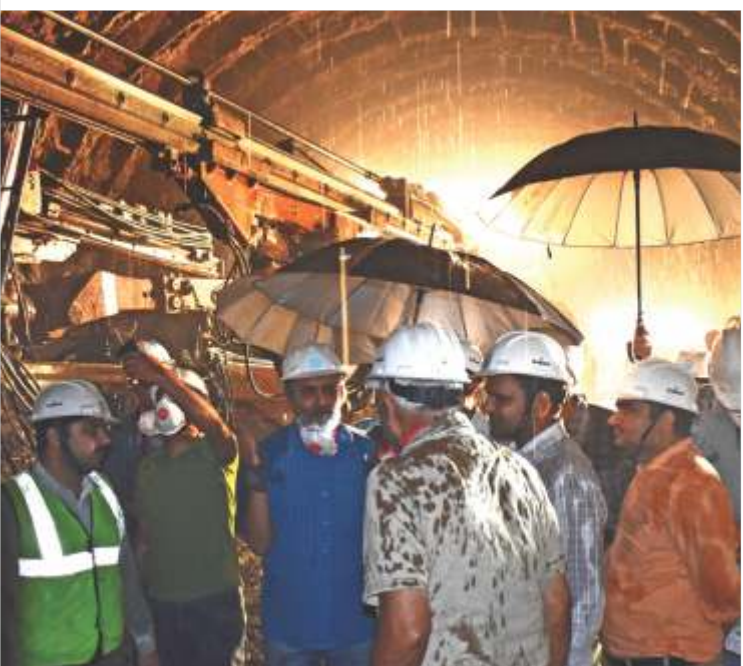
Note the seepage of water and the need for umbrellas
