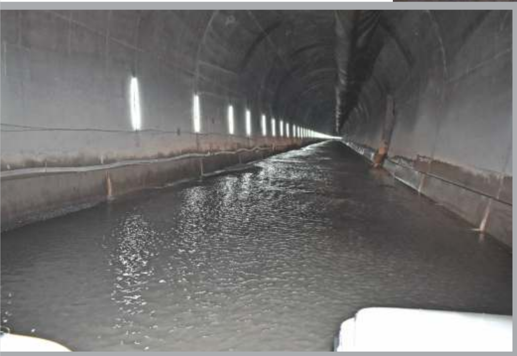
Water gushing down Tunnel No. 5
