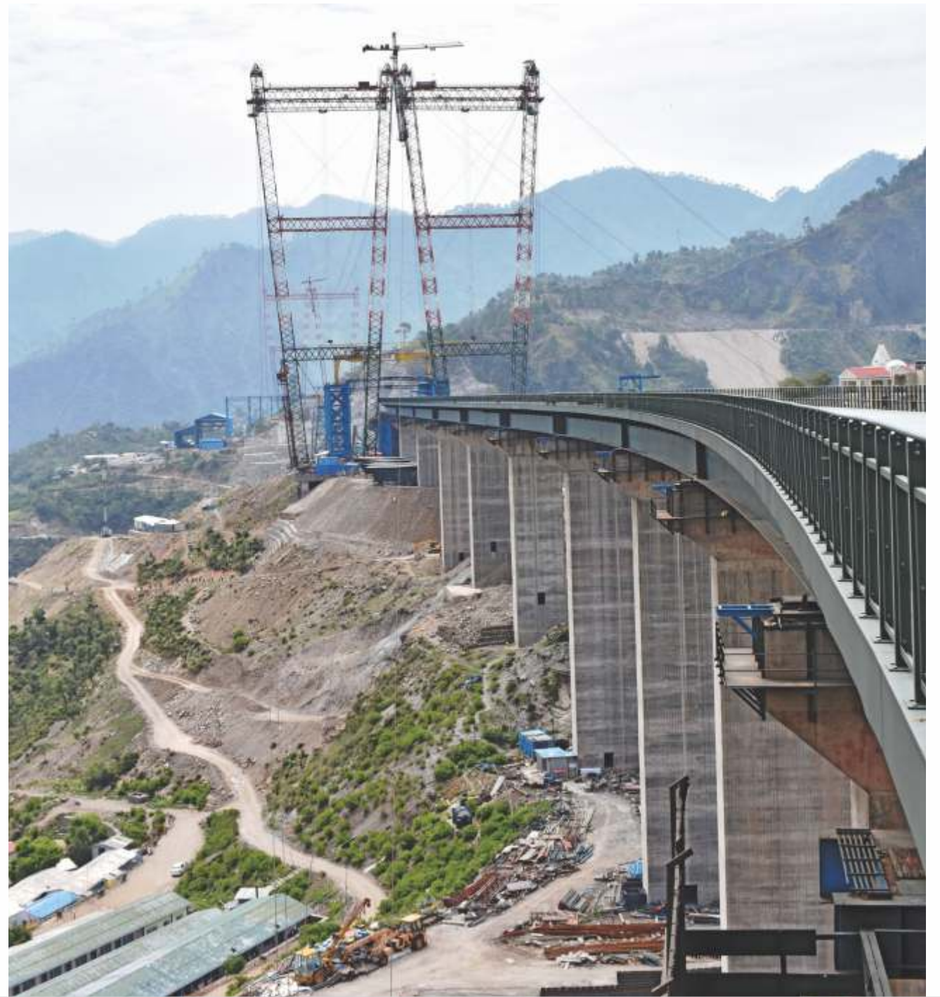
End of the curved viaduct. Steel pylons for the travelling crane are at its end
