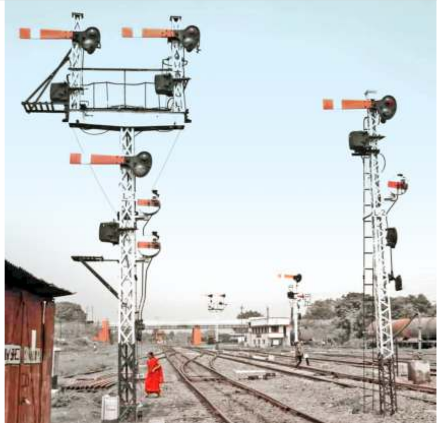
Semaphore signals that are now being replaced by colour light signals
