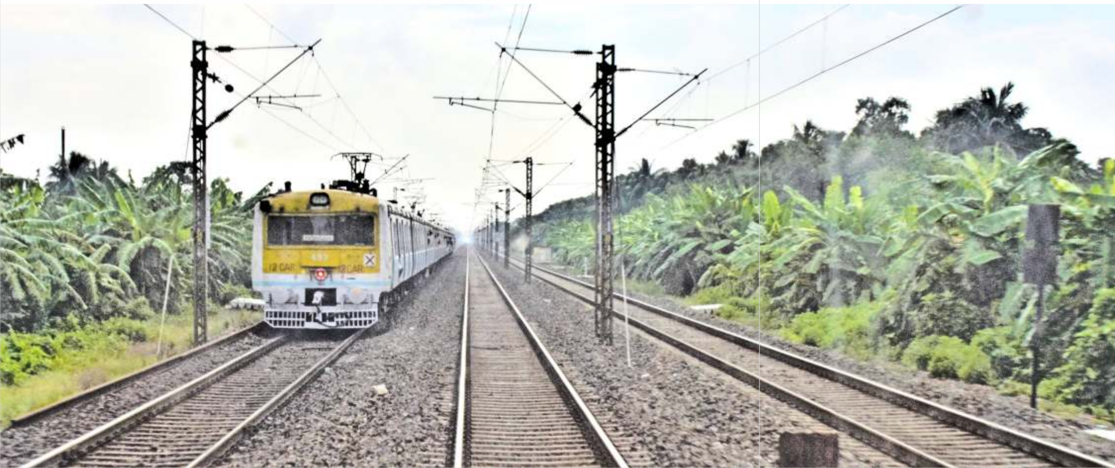
Electrified rail track between Howrah and Kharagpur. A 12-car EMU can also be seen
