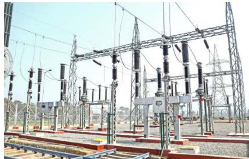
A view of the sub-station
